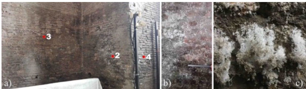
Figure 72 (a) Points of the masonry inside the Hall I where the samplings were made (b) Detail of the masonry and (c) of the salt efflorescences.
