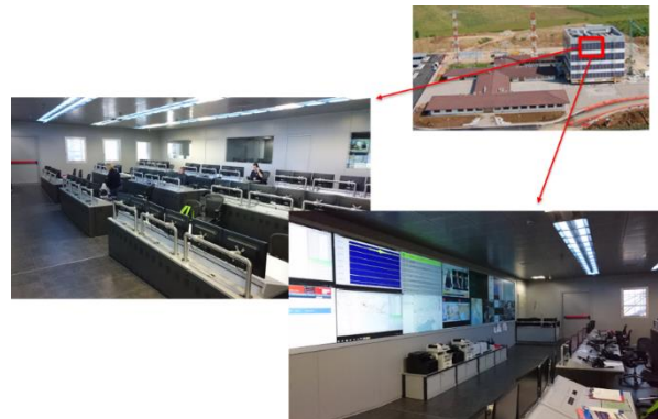
Figure 4: Operations room (large)
